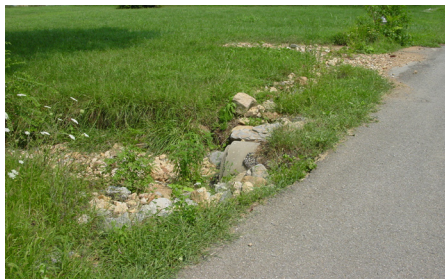
Stormwater drainage and curb and gutter issues along Ray Road
