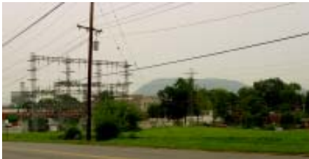
Power station along Salem Avenue
